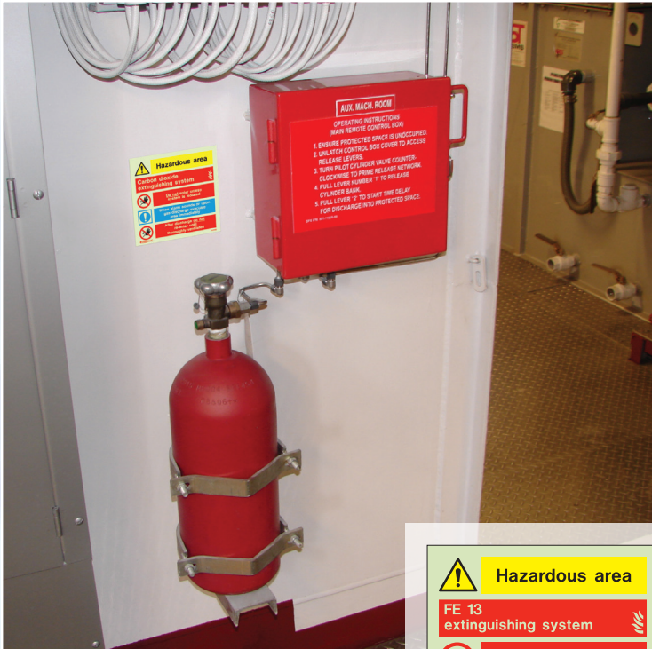
6516E (Hazardous area, carbon dioxide extinguishing system)
